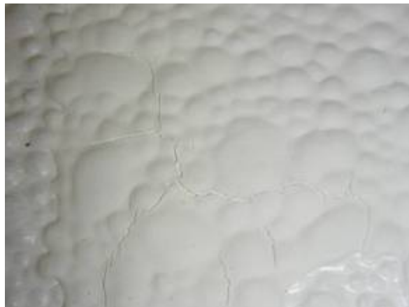
Cracking in decorative paints
